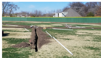
McDonald Stadium Irrigation
