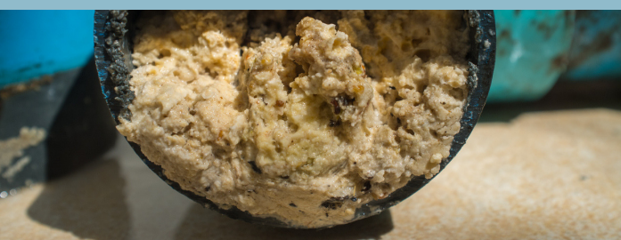
Grease is a frequent cause of sewer blockages/backups.
