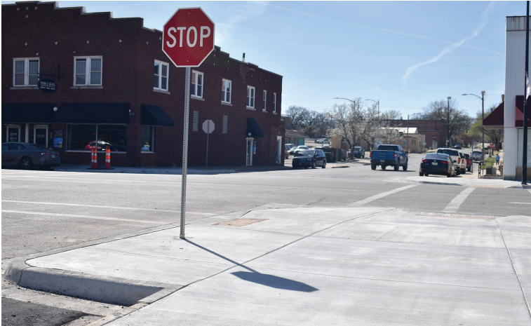
The bump outs at First and Main streets were completed in March. This project extended the curb and crosswalks to allow better visibility for pedestrians crossing the street. Additional bump outs are being constructed at Pine and Main.
